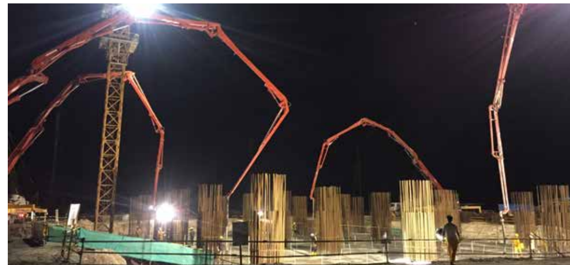
四蛟龙齐助尼日利亚建设 Four boom pump are cooperating like dragons in Nigeria
