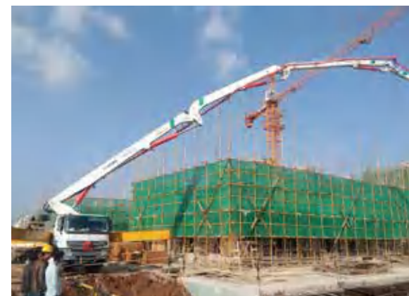
徐工HB52V泵车云南施工 XCMG HB52V boom pump is working in Yunnan
