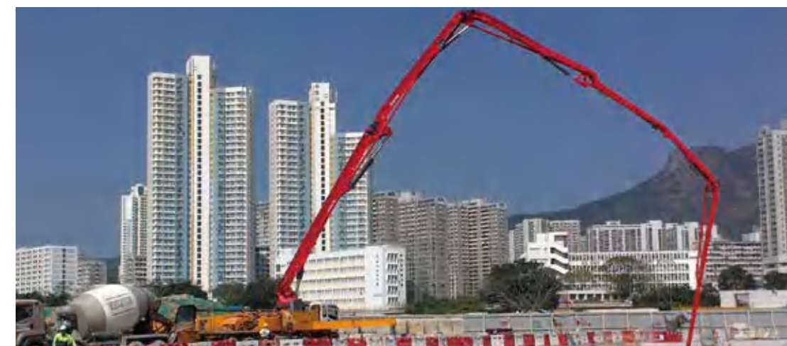
HB53K泵车香港地铁站小试牛刀 First show of HB53K boom pump at subway station of Hongkong
