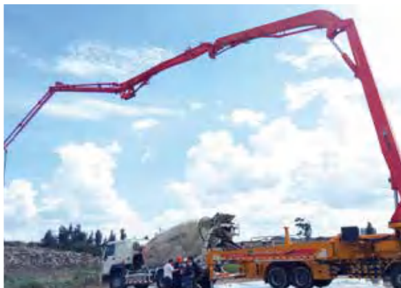
徐工泵车助力埃塞俄比亚建设 XCMG boom pump is working in Ethiopian construction
